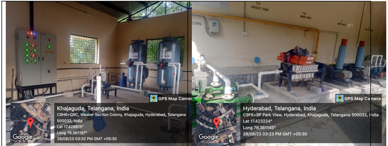
100KLD Electrolyte type Sewerage Treatment Plant -02
